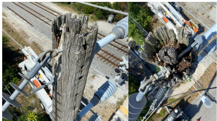
Figure 8 Rotted power poles present dangers to the community and when they fail will cause an outage.
